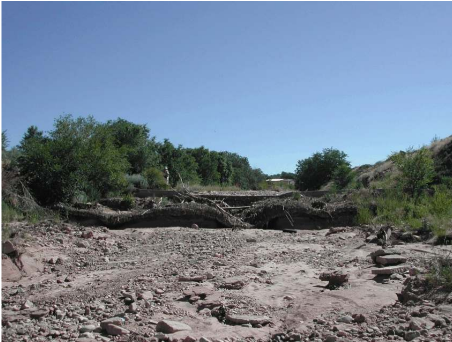
Figure 49. Grade control structure GCS-7, downstream from Camino Carlos Rael, showing failure of the erosion control apron and undermining of the structure. View is upstream. Photo by J. Pittenger, 26 June 2007.
