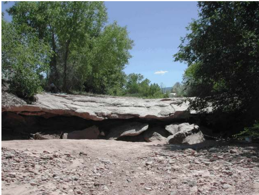
Figure 22. Grade control structure GCS-5 at the Vereda de San Antonio crossing. View is upstream. Photo by J. Pittenger, 26 June 2007.
